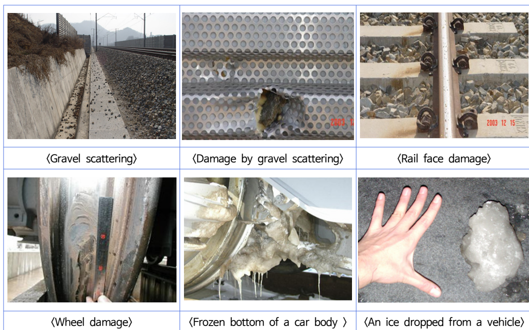
Figure 63 | Problems of Ballast Track of Gyeongbu HSR Phase 1 (Seoul~Daegu)
